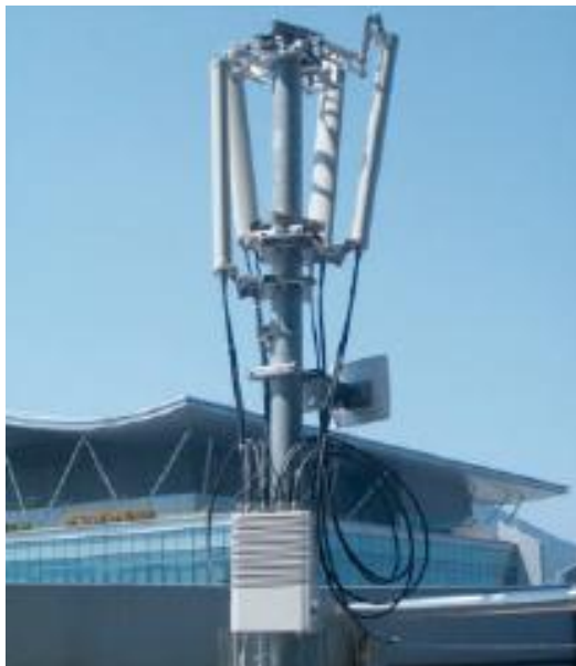
Figure 2: Altai A8 WiFi Cellular Base Station with Standard Smart Antenna
